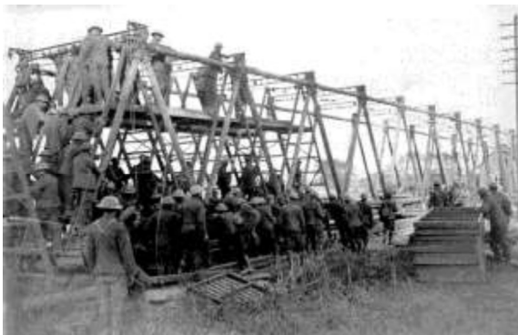
Figure 4: Building the Inglis Mk II Bridge over the Canal du Nord at Marquion, France, in 1918.
