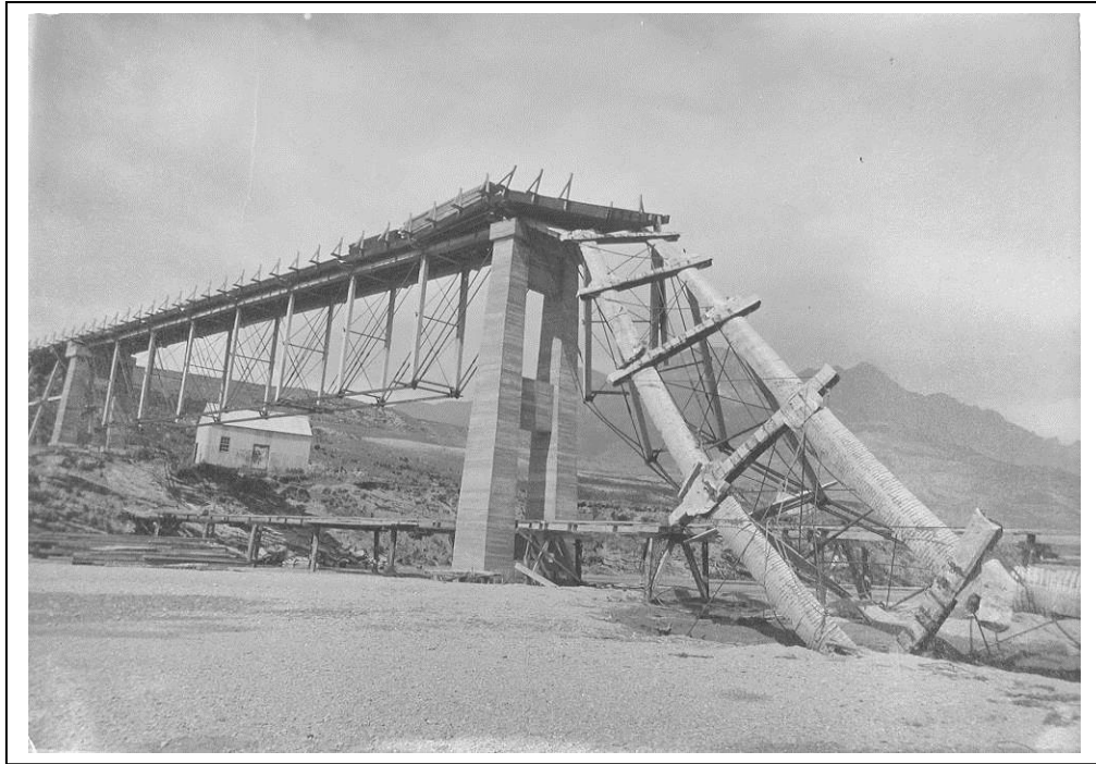
Lower Shotover Bridge. showing pier that collapsed during construction in 1911 [?]. Lakes District Museum collection, EL0025.
