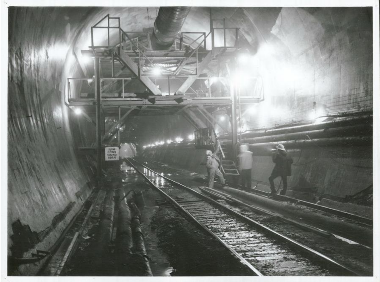
Above: Workers use a “jumbo” to inspect the lining of the tailrace tunnel, August 1967. Archives New Zealand, R24730671, photographer: Mr Neill.
