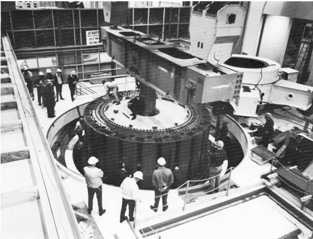
Above: West Arm Powerhouse. Generator No.5 – positioning rotor in stator. October 1970. Photo reference HA2394. Meridian.
